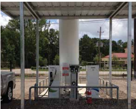
Above ground vertical tank installation
