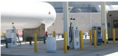
Above ground horizontal tank installation
