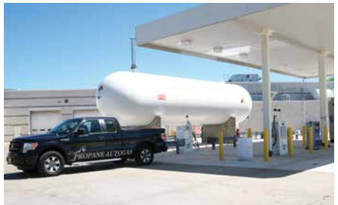
Above ground horizontal tank installation
