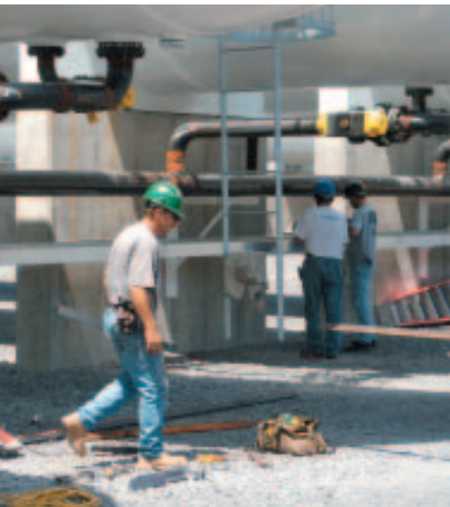
Electricians run conduit across the concrete piers that support the hulking propane storage tanks.
