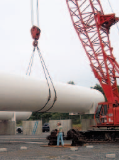
A special crane capable of lifting 300 tons is used to unload and install the 90,000-gallon storage tanks, each of which weighs 150,000 pounds.
